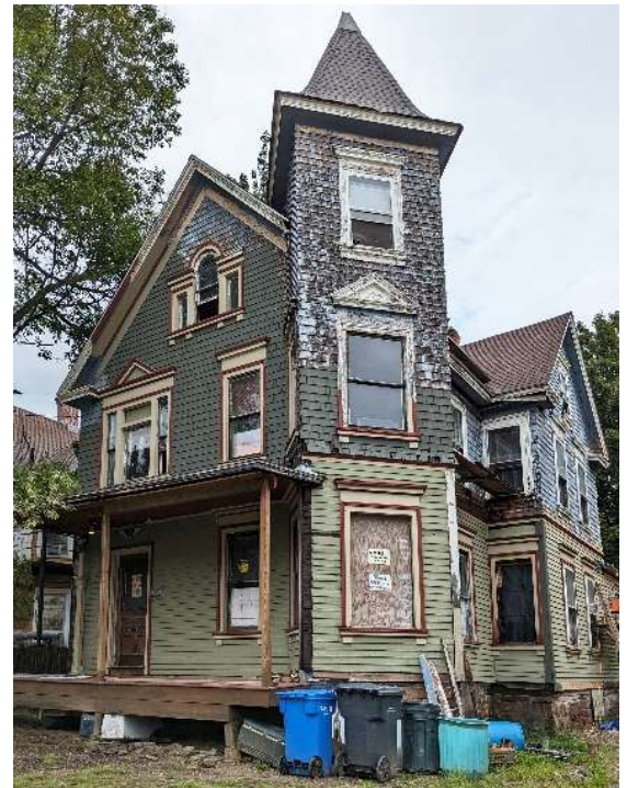
32 Girard in 2023:Mid-project, showing condition of shingles on the 3rd floor and new paint on the front.
