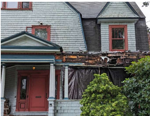
146 Kenyon, porch failure 2023
